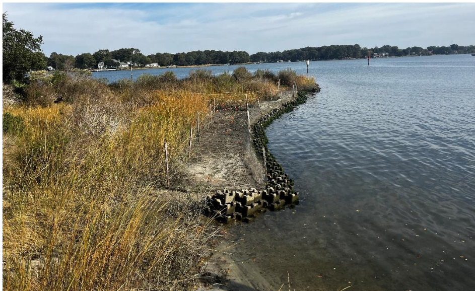
This restoration at the mouth of Knitting Mill Creek incorporates oyster structures and wetland grasses to provide habitat and erosion protection.
