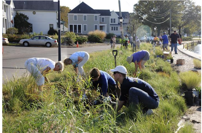
Partners including Lafayette Wetlands Partnership, the City of Norfolk and Elizabeth River Project planted native salt-tolerant grasses and flowers along Mayflower Road.
